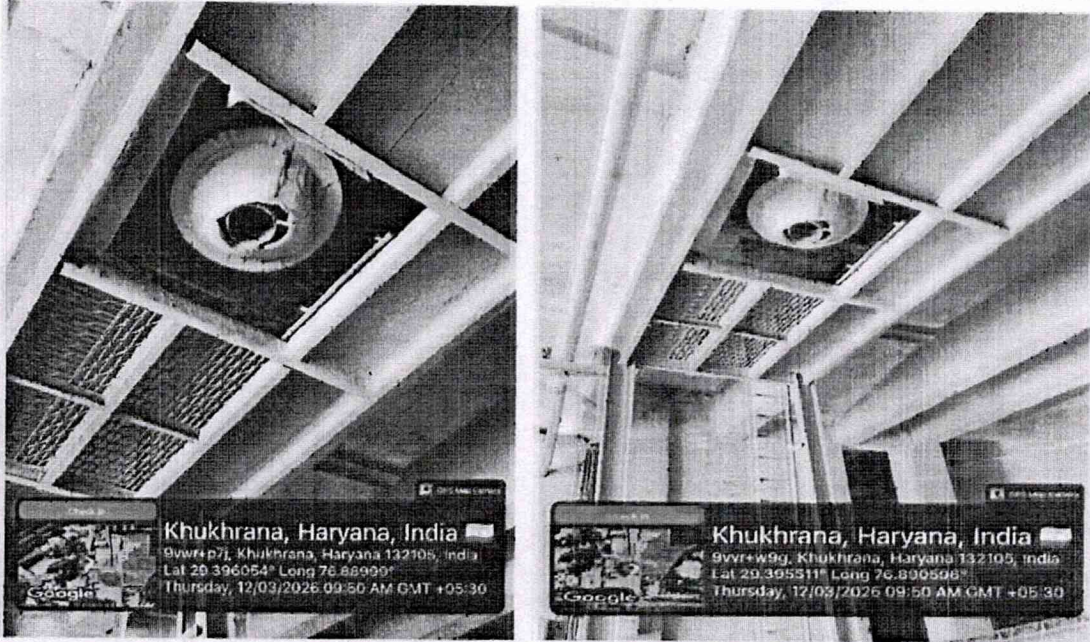
Annexure :-VII Telescopic Chute at Cement Bulker Loading section
